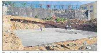
The site where villas are being constructed at Katra in Reasi district of Jammu and Kashmir.
